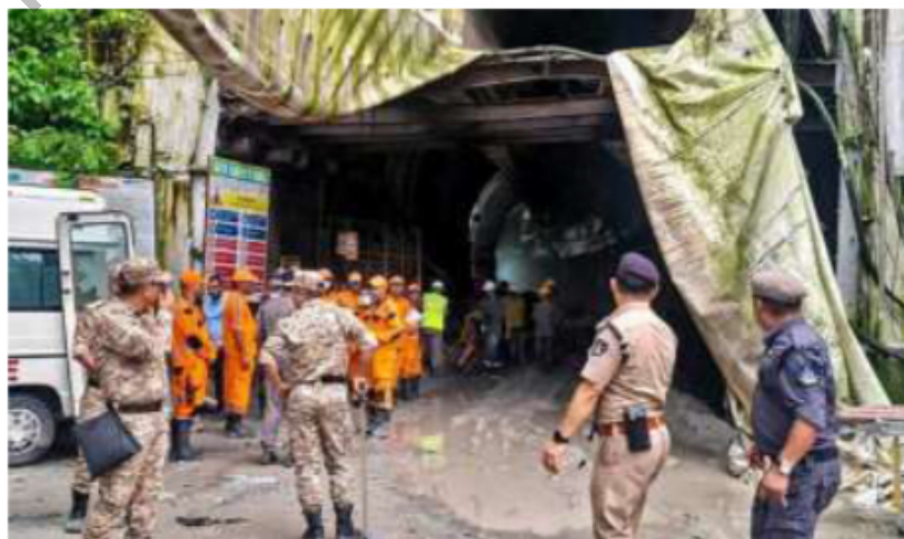
Police and rescue workers at the under-construction tunnel that was damaged in a blast in Sikkim's Namchi district on July 20. PTI
