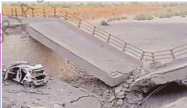
The damaged portion of a bridge in Bandar Khamir, Hormozgan province of Iran, Friday, REUTERS
