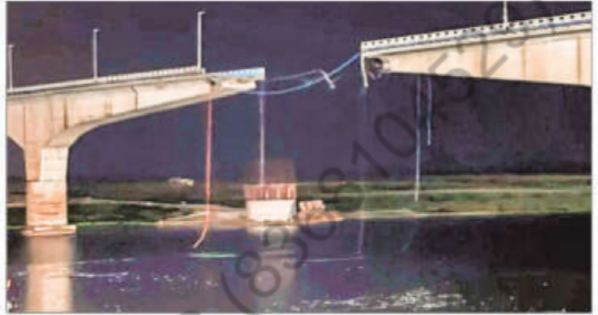
The partially damaged Vikramshila Setu in Bhagalpur on Monday. PTI
