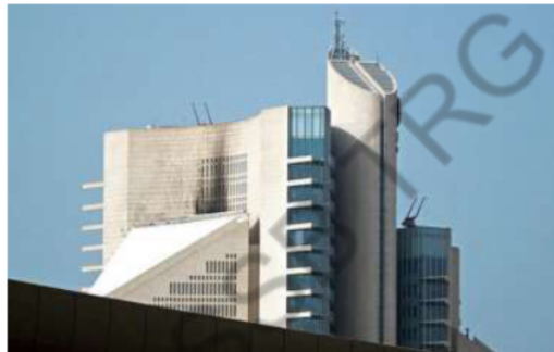
Material damage: The impact of a fire caused by a drone attack on a building of the Kuwait Petroleum Corporation on Sunday. AFP
