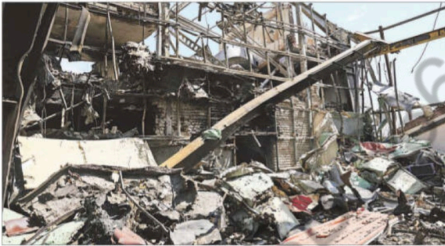
The research building of the Shahid Beheshti University, which was damaged by a strike, in Tehran, on Saturday. REUTERS
